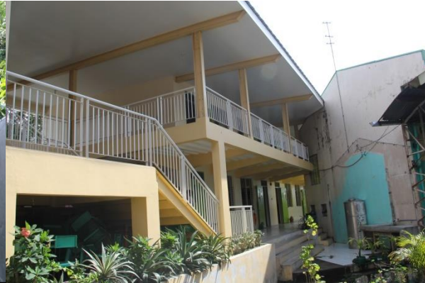
Lack of space between PSIP building and existing building in Taykin Elementary School
